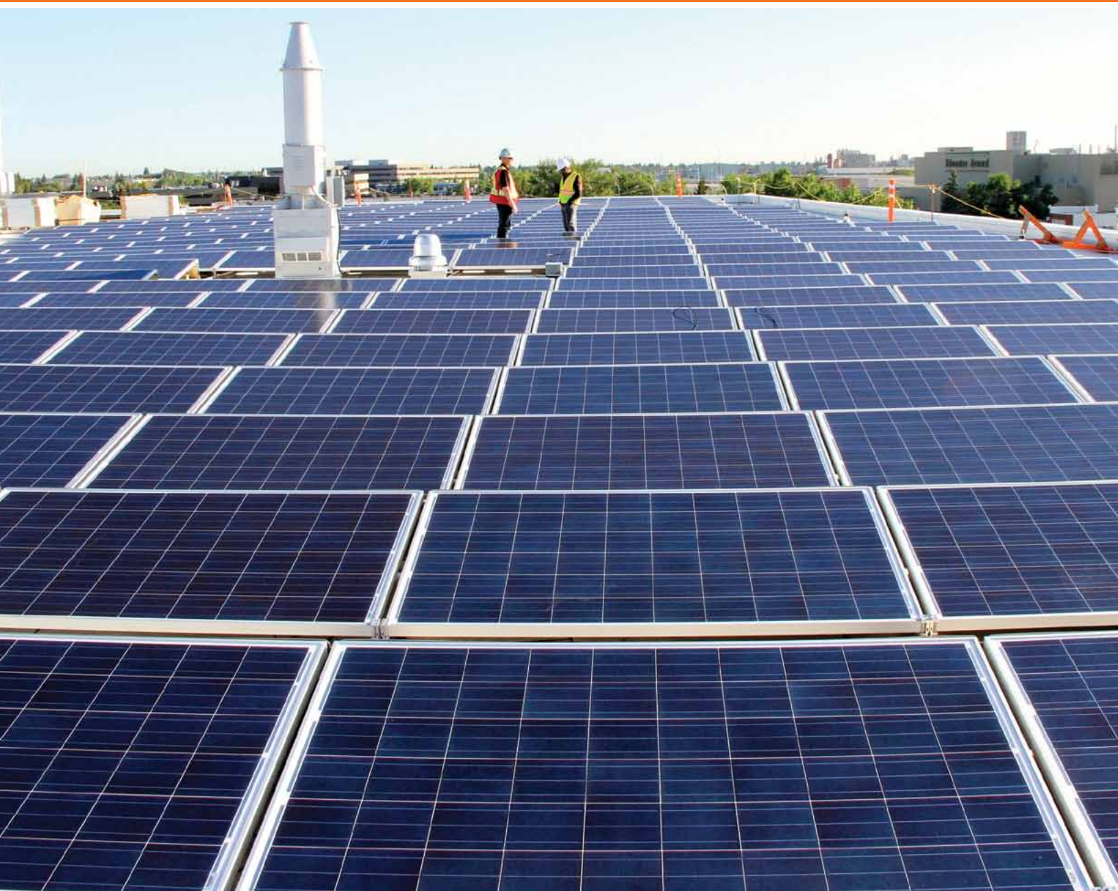
Photo: Solar array in Edmonton, Alberta.
