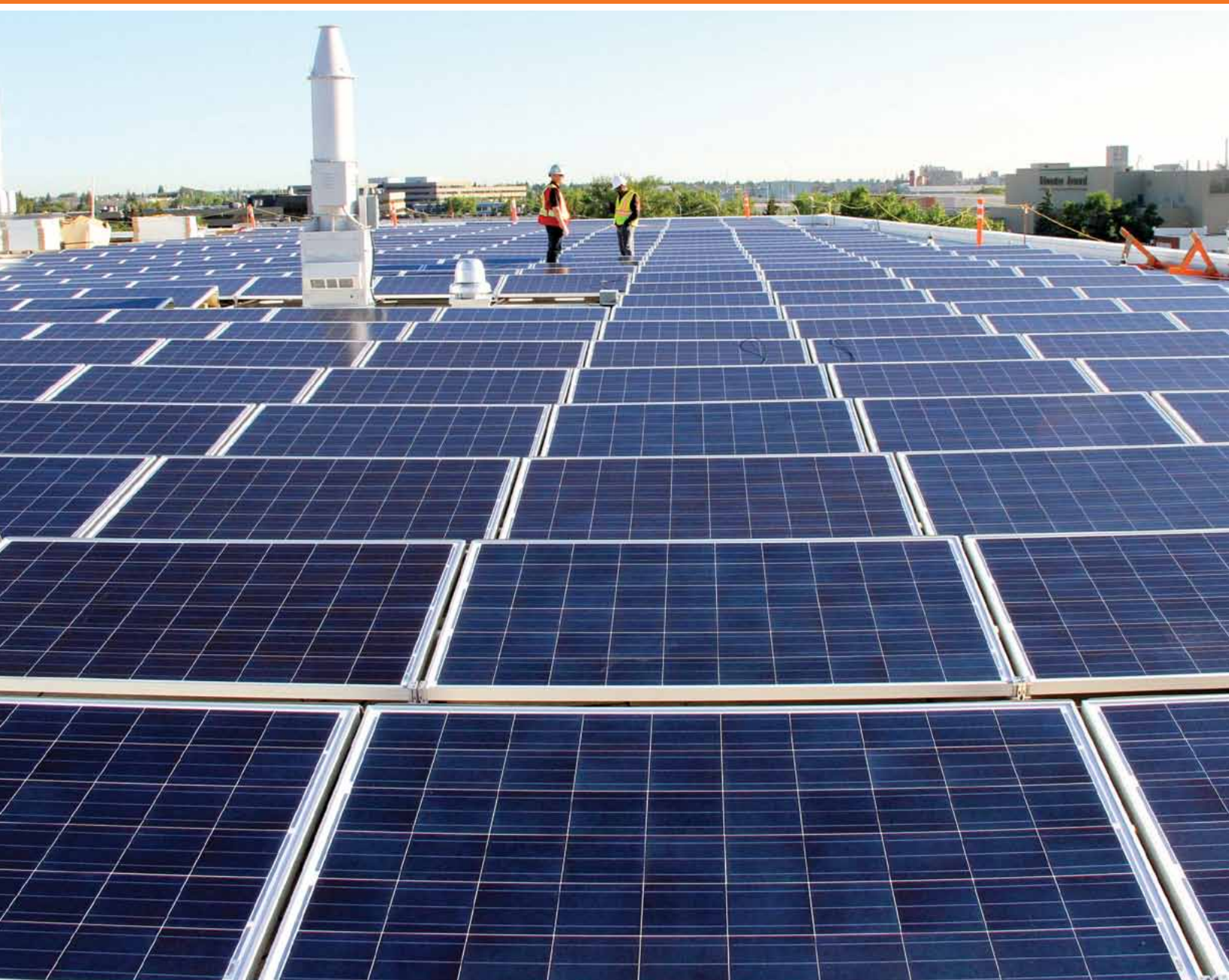
Photo: Solar array in Edmonton, Alberta.
