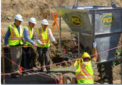
Left: Workers pour concrete at a new hospital and health centre in Burns Lake, B.C. Photo courtesy of B.C. Northern Health Authority.
