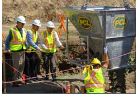
Left: Workers pour concrete at a new hospital and health centre in Burns Lake, B.C. Photo courtesy of B.C. Northern Health Authority.
