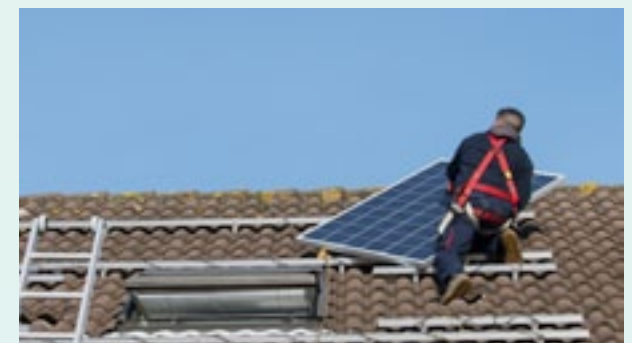
Rooftop solar installation
