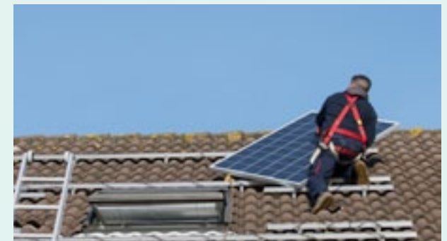
Rooftop solar installation
