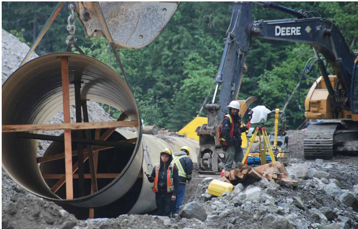
First Nations workers assemble a section of penstock for the Kwoiek Creek run-of-river hydroelectric project. Photo: Innergex Renewable Energy.
