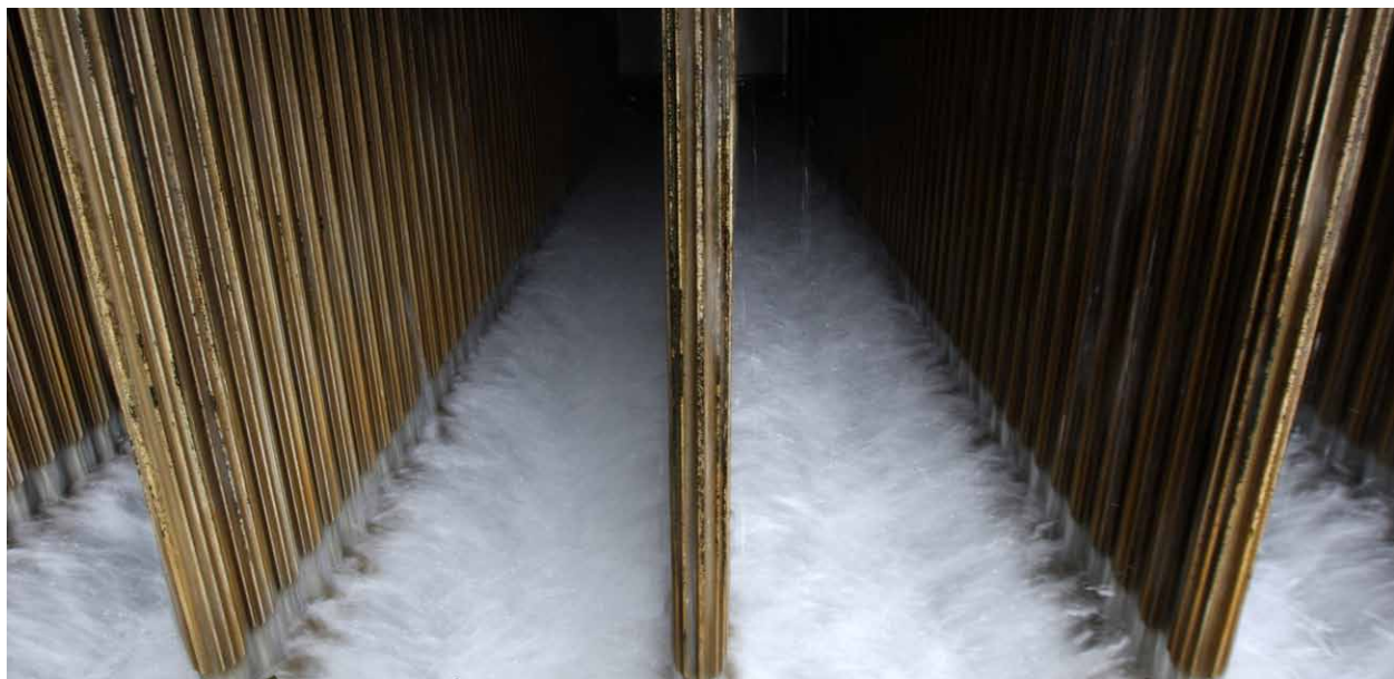
Sea water flows in an open rack type liquefied natural gas (LNG) vapourizer at Tokyo Gas Co.'s Sodegaura plant in Sodegaura City, Chiba Prefecture, Japan. Photo: Getty Images.
