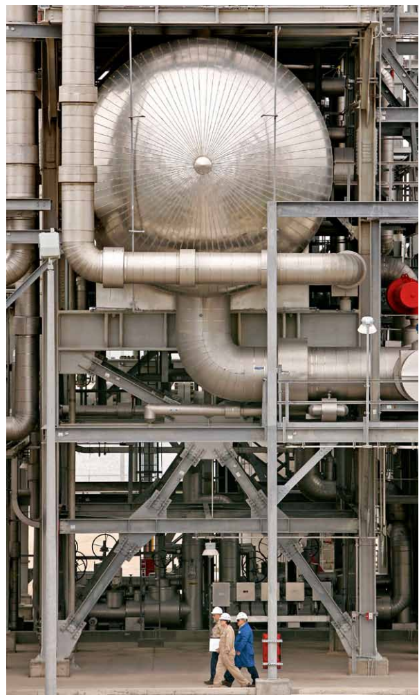
The vapourizer at Freeport LNG in Quintana, Texas. Photo: Getty Images.
